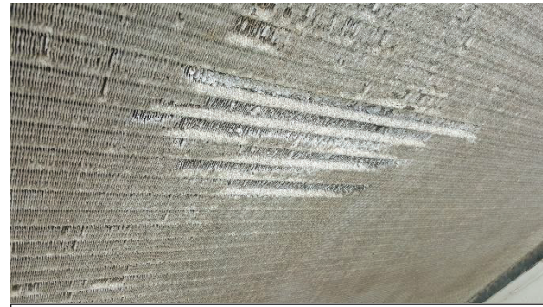
Photograph #8 – Damaged Condenser Coil Fins
