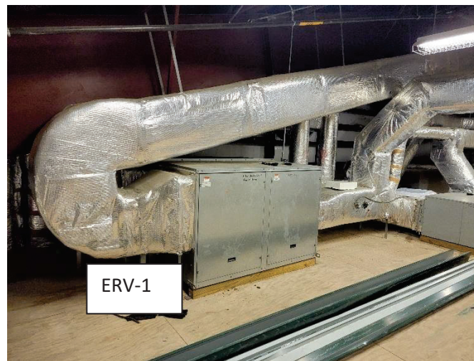
Photograph #11 – Energy Recovery Ventilator-1
