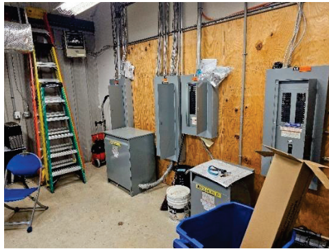
Photograph #18 – Electrical Gear in 2014 Addition
