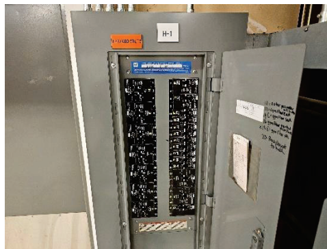
Photograph #16 – Typical 480Y/277V Branch Panelboard
