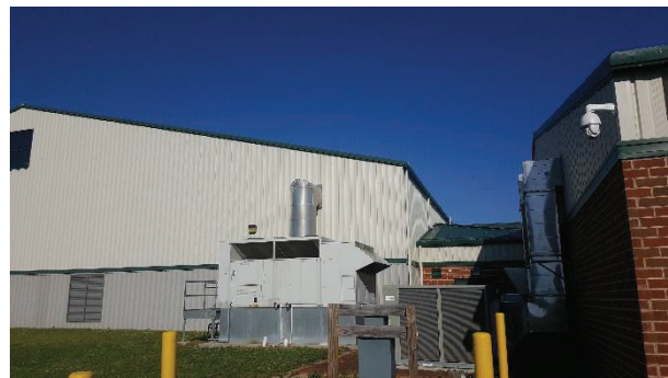
Photograph #2 – Existing RTU #2
