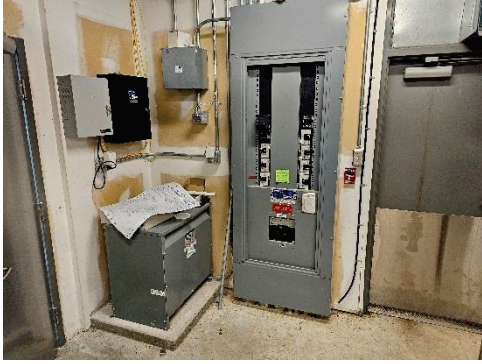
Photograph #14 – Main Distribution Panelboard
