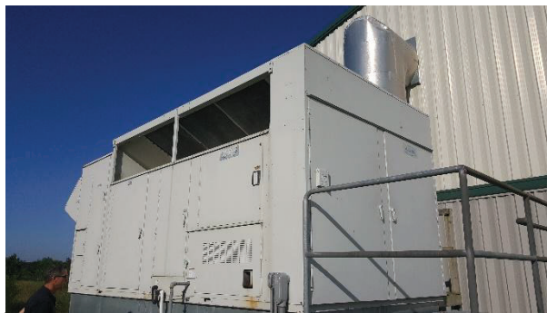
Photograph #1 – Existing RTU #1
