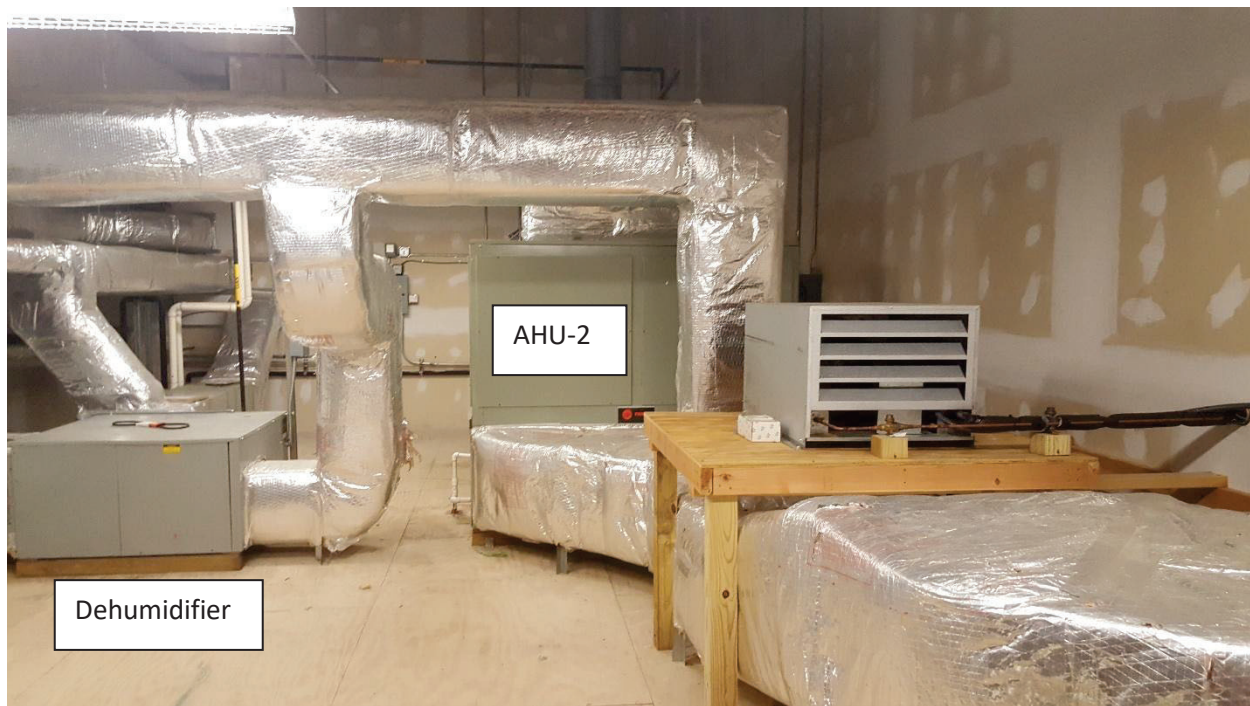
Photograph #10 – AHU-2 and Dehumidifier
