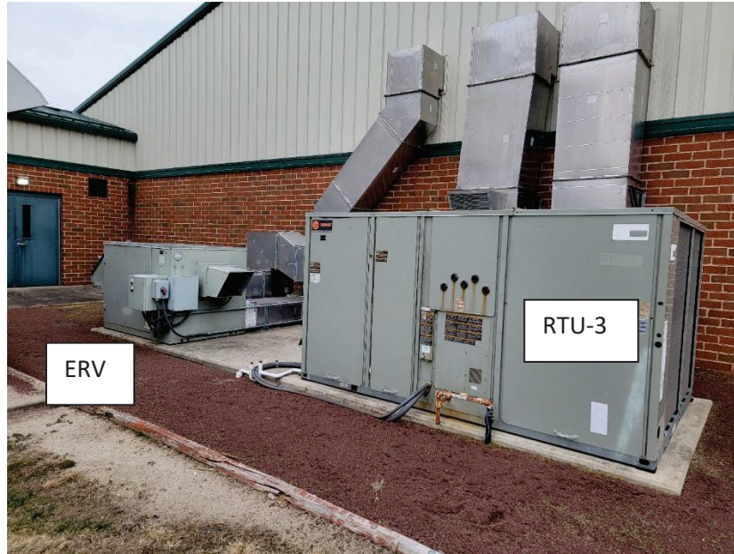
Photograph #12 – RTU-3 and ERV Serving 2014 Addition
