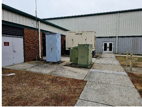
Photograph #19 – Generator and Automatic Transfer Switch
