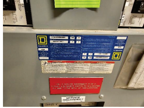
Photograph #15 – MDP Nameplate
