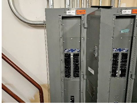
Photograph #17 – Typical 208Y/120V Branch Panelboards
