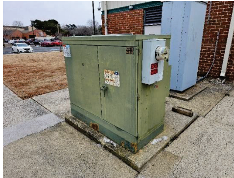
Photograph #13 – DPL Transformer with CT Metering
